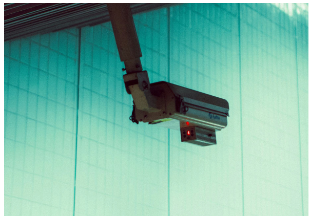
CCTV Cameras in Beijing, China
